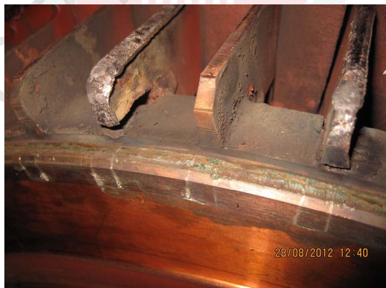
Figure 2.1: Two broken rotor bars at the end rings [21].
